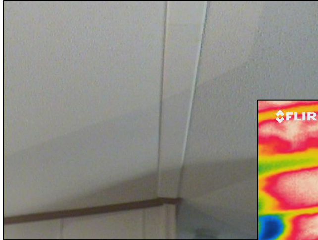
Missing ceiling insulation
